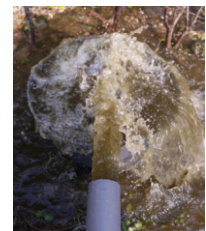
Backwash discharge sewage
